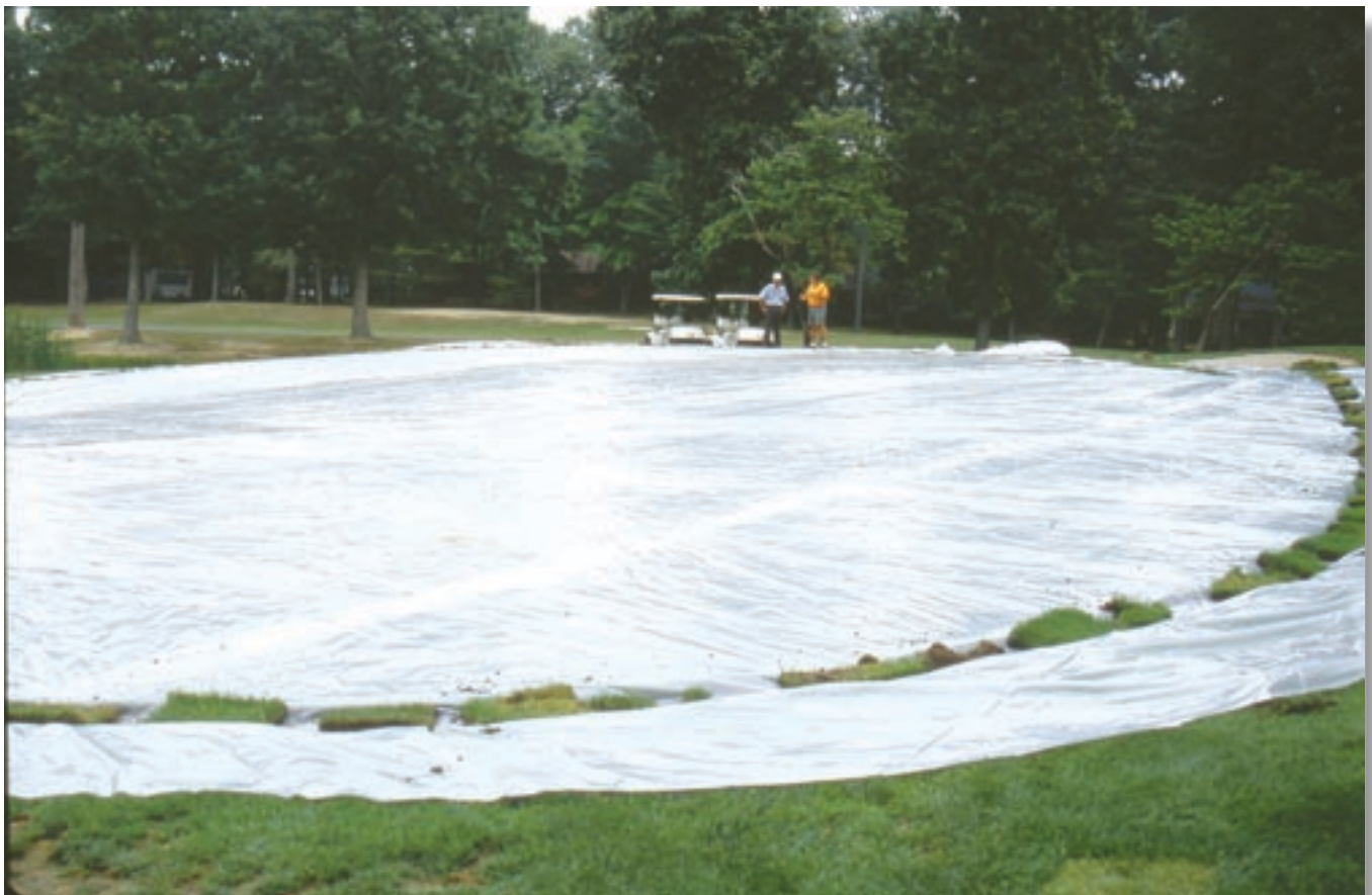
Figure 4. Sod strips cut from the periphery of the green were used to seal the plastic tarps that covered the green following Basamid application.
